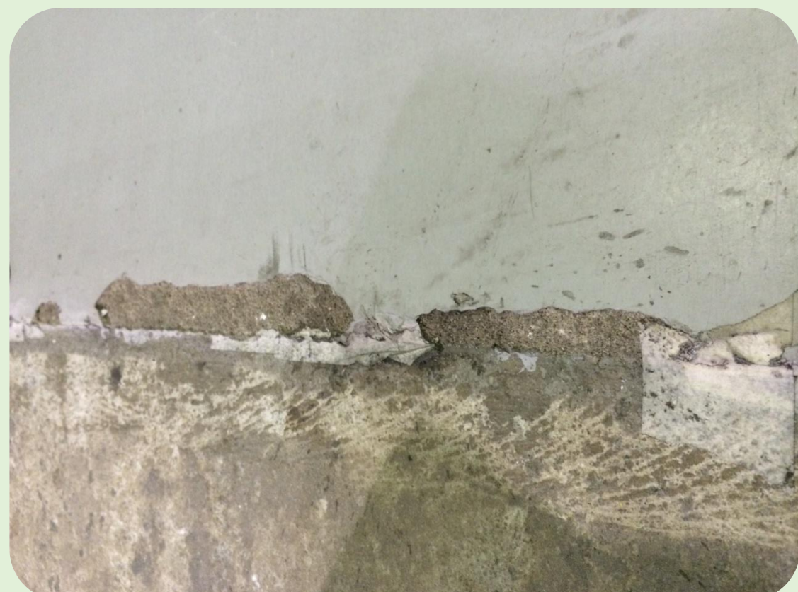
Before: Cracks and holes of flooring that can caught the wheels and cause vessels to topple.
