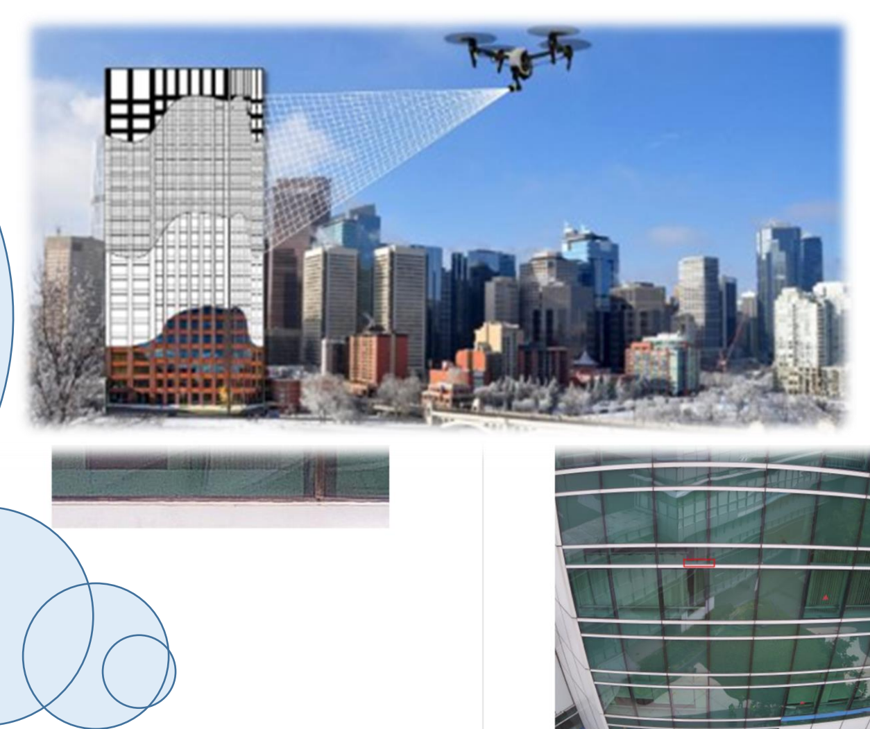
Defect Type - Worn off rubber gasket Severity - Require Repair Details - Worn off rubber gasket Resolution - Replace the rubber gasket and ensure the water and air tightness.
