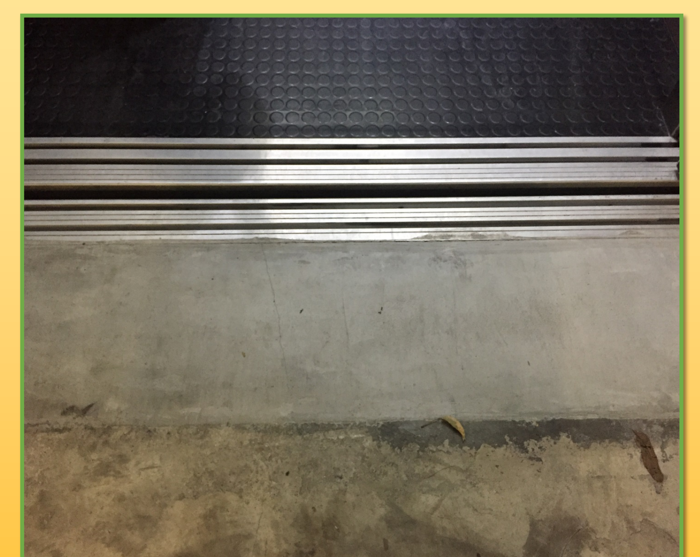
Height difference between the lift landing and lift door frame evened out.
