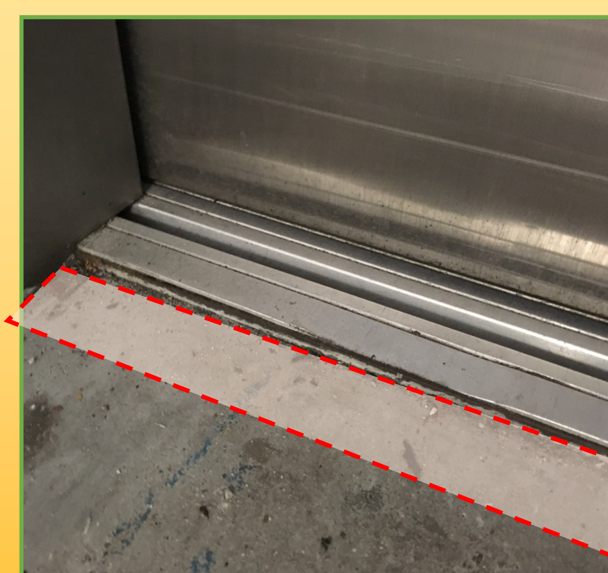
Proposal to level the lower lift landing with a slope extending from the door frame.
